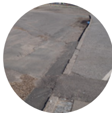
Poor ground condition
