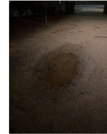
Fig.31 Photo of water accumulation on unpaved path near entrance.
