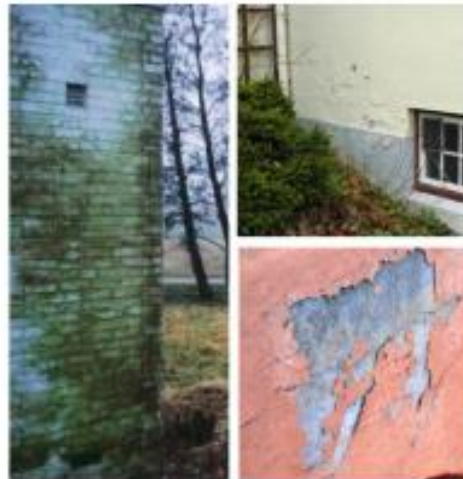
Examples of visually apparent moisture induced damage of external facades.
