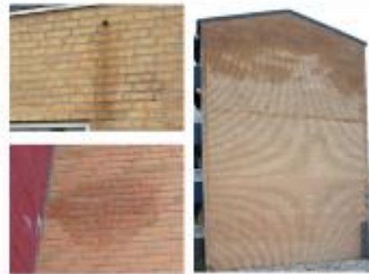
Examples of stains and wet spots: their break on rendered masonry facade, wet spots on masonry facade, local defects causing concentrated moisture accumulation. Moisture accumulation at top of facade gable, likely due to precipitation.
