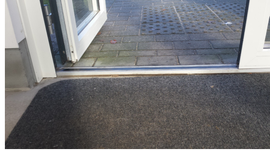
III. 6. Doorstep at an exit door
