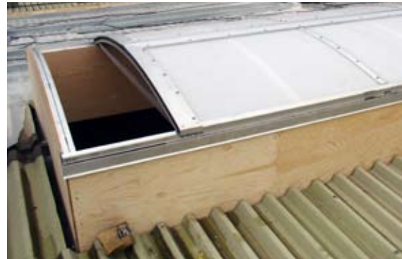
[ 23 ] The procedure of mounting the motors and opening modules goes on down towards the last end gable until the lightrow consists of mounted opening modules with spaces in between for fixed pc plates.
