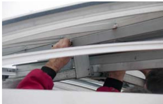
[ 17 ] The motor is activated slightly to ease the mounting of the motor brackets to the receiving brackets on the two opening module.
