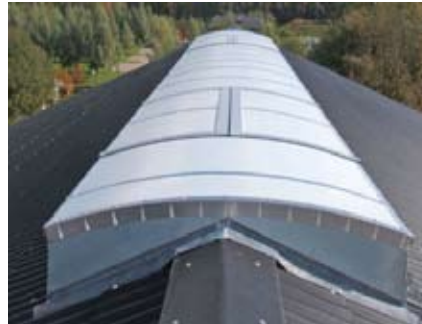
Vaulted PC lightrow with fire ventilation mounted on a ridge tile roof.
