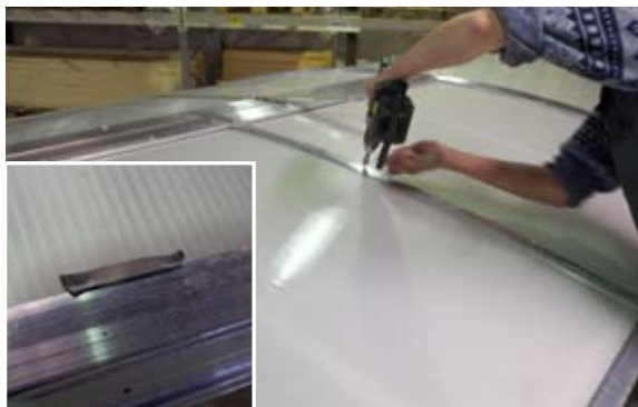
[ 22 ] In the middle of the opening modules, alu profiles with underlying weather strips are mounted to an underlying brace. Extra weatherstrip in top and bottom.
