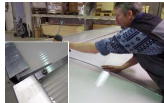
[ 18 ] Silicone filler is applied around the alu profile [ 17 ] in top and bottom to prevent water from getting in and moving inside through the holes for the screws.
