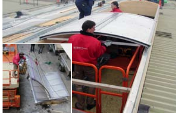
[ 11 ] An opening module and a motor is hoisted into the lift. The opening module is placed loosely on the two side frames.
