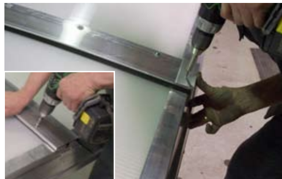
[ 23 ] An alu profile with self-expanding weatherstrip is mounted where the opening and fixed modules meet and fixed to the opening module to weather seal this area.
