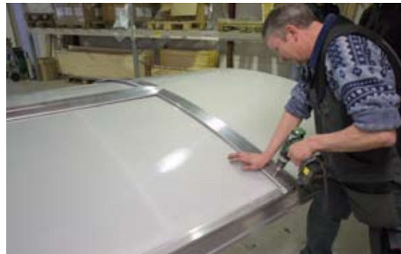
[ 20 ] The alu profiles from [ 19 ] is mounted onto the opening modules of the skylight.
