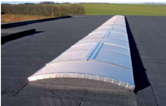
[ 25 ] Here the lightrow is completed with a new felt roof. (Reference photo)
