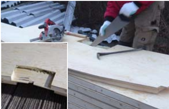
[ 4 ] The second person from the mounting crew performs the modifications to the frame if it is needed.
