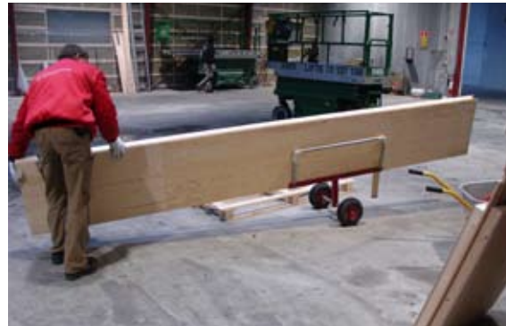
[ 5 ] The modules for the wooden frame are transported into the building below the hole for the lightrow on a wagon for easier handling.
