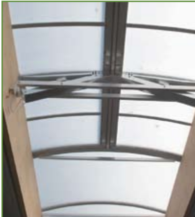
ill. 3.80 - Domex light row from the inside.
