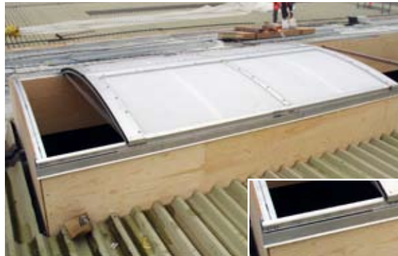
[ 14 ] The opening module is placed in its correct position using alu profiles that ensures the correct distance to the end gable.
