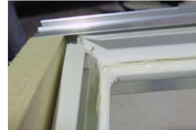
Applying construction glue to make the corner between the condensation profiles tight.
