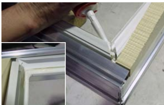
[ 13 ] Construction glue is filled into the gap between the plastic condensation profiles and distributed to make the corner water tight.
