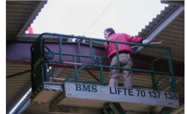
[ 3 ] One of the two people from the mounting team measures the hole to identify if anything should be cut away for the wooden frame to fit into the hole.
