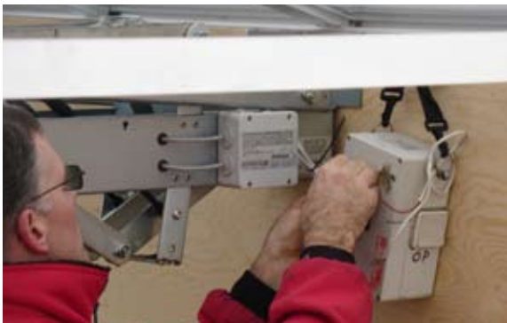
[ 16 ] The motor's electrical system is connected to a 24V portable battery case with controls for opening/closing.
