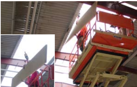
[ 7 ] The end gable is lifted into place using an electric winch mounted to the work lift.
