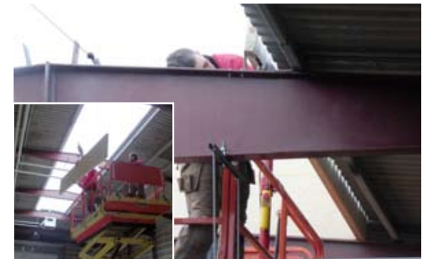
[ 9 ] The mounting crew mounts angle brackets on the next bearing steel structure and mounts a side frame. This continues all the way to the end and the second end gable is mounted.
