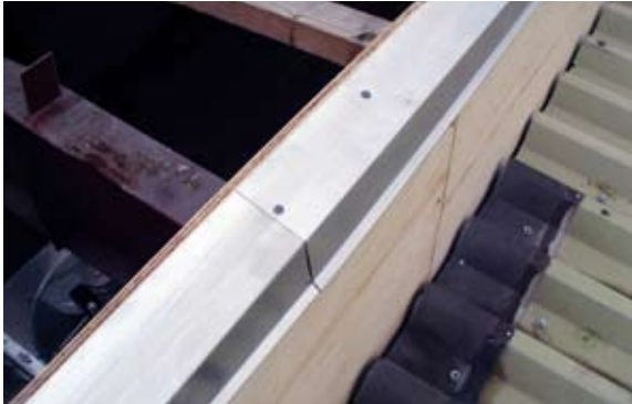
[ 10 ] Alu profiles that lead water away from the top of the side frames are mounted. Felt roofing will be burned onto the side gables up under the alu profile.
