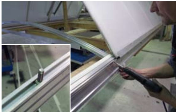
[ 10 ] Bolts are slid into the side of the transverse braces, and a transverse brace is mounted on each side of the opening modules.
