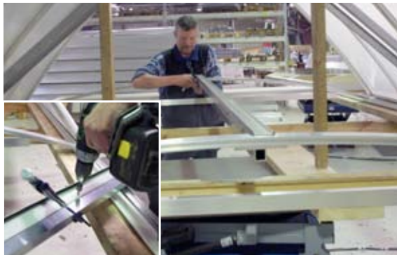
[ 11 ] A plastic profile to collect condensation is mounted on an alu brace that is mounted between the bolts in the two transverse braces shown in [ 10 ].
