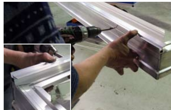
[ 6 ] Alu profiles to fasten the fixed PC plates onto, are mounted to each long side on each side of the opening modules.
