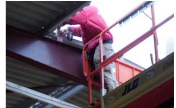
[ 6 ] Angle brackets to fix one end gable are mounted onto the bearing steel construction.
