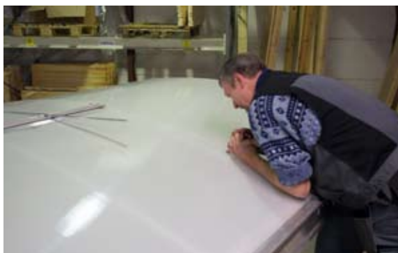
[ 16 ] The gap between the fixed PC plates and the opening modules are checked for the required clearance. Potential surplus material is cut away.
