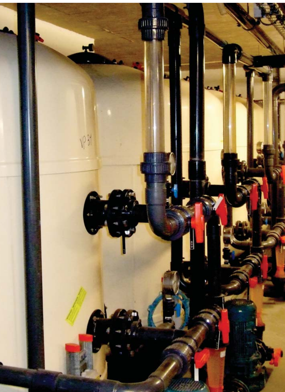
Swimming pool Haraldslund. Basement. Photo. An extensive infrastructure of technical equipment ensures fresh clean water and air to the above pool area. The extents of this secret underworld almost match the public world above.
