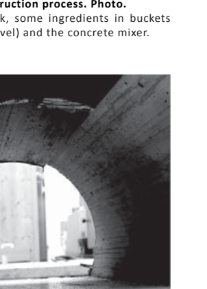
Cast concrete. Photo. The formwork is removed to reveal the inside structure of the cast.
