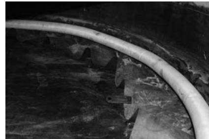
Figure A.11: The fire hose pressing the rubber band and the skirt against the tank side.
