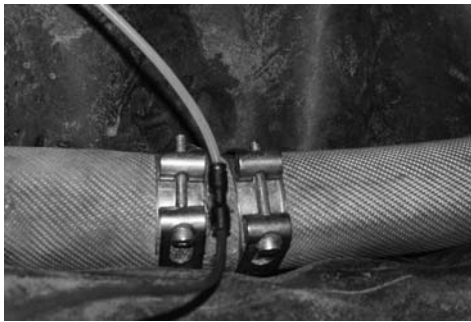
Figure F.3: Fire hose with old joint.
