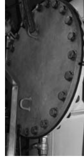
Figure 7: The openings in the tank hermetically sealed.
