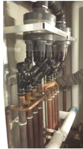
Drain water heat exchanger
