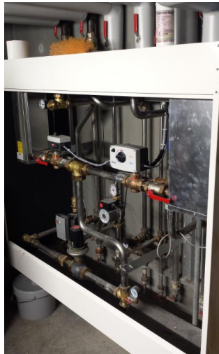
Plate heat exchanger connected to District Heating
