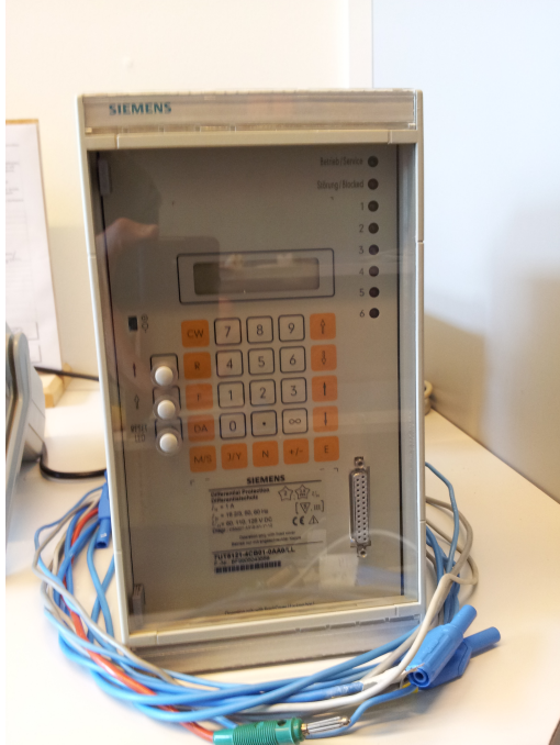
Figur 7.3. Viser differentielrelæet: SIEMENS SIPROTEC V3.0 - 7UT5121-4CB01-0AA0/LL (forfra).
